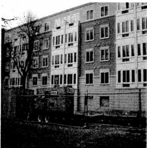
Nearly complete Capper II units.
